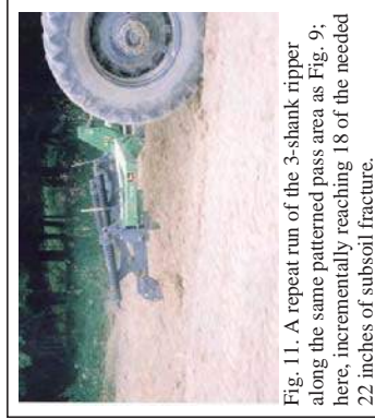
Fig. 10. An early pass with a 3-shank deep ripper penetrating only 8 inches into this worksite's severely compressed subsoil.
