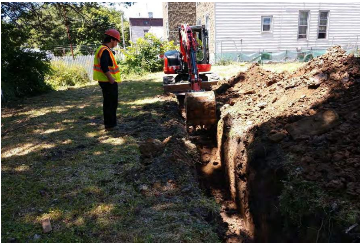
Photo 6: Trench 3 was excavated in the northern portion of the APE. View to the west.
