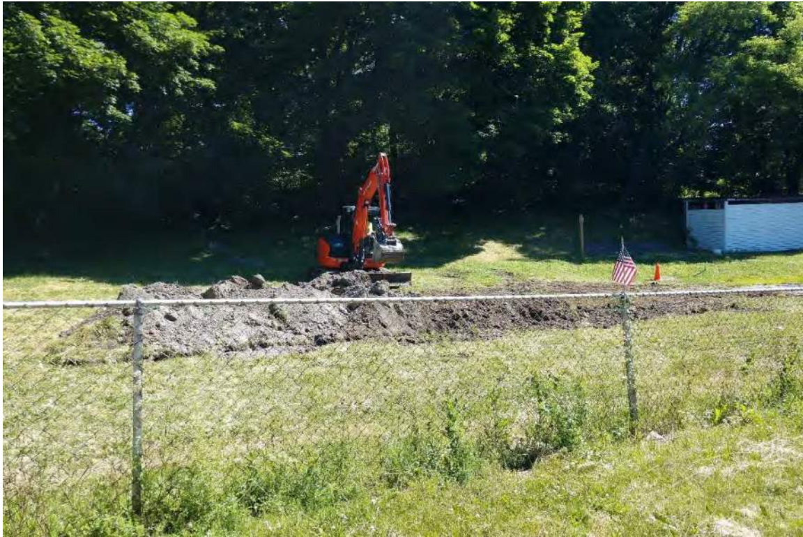
Photo 2: All trenches were backfilled upon completion. View to the north from Scott Street.
