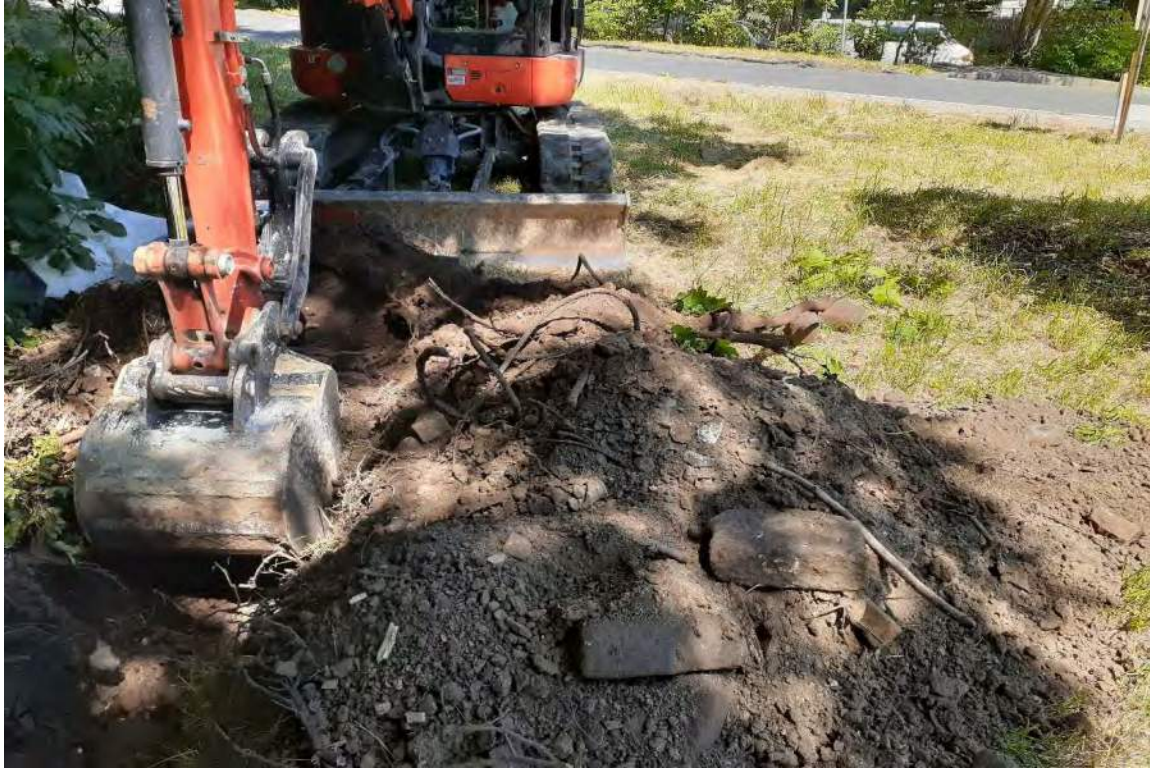
Photo 10: The upper level of Trench 5 consisted of fill that contained metal and brick. View to the northeast.
