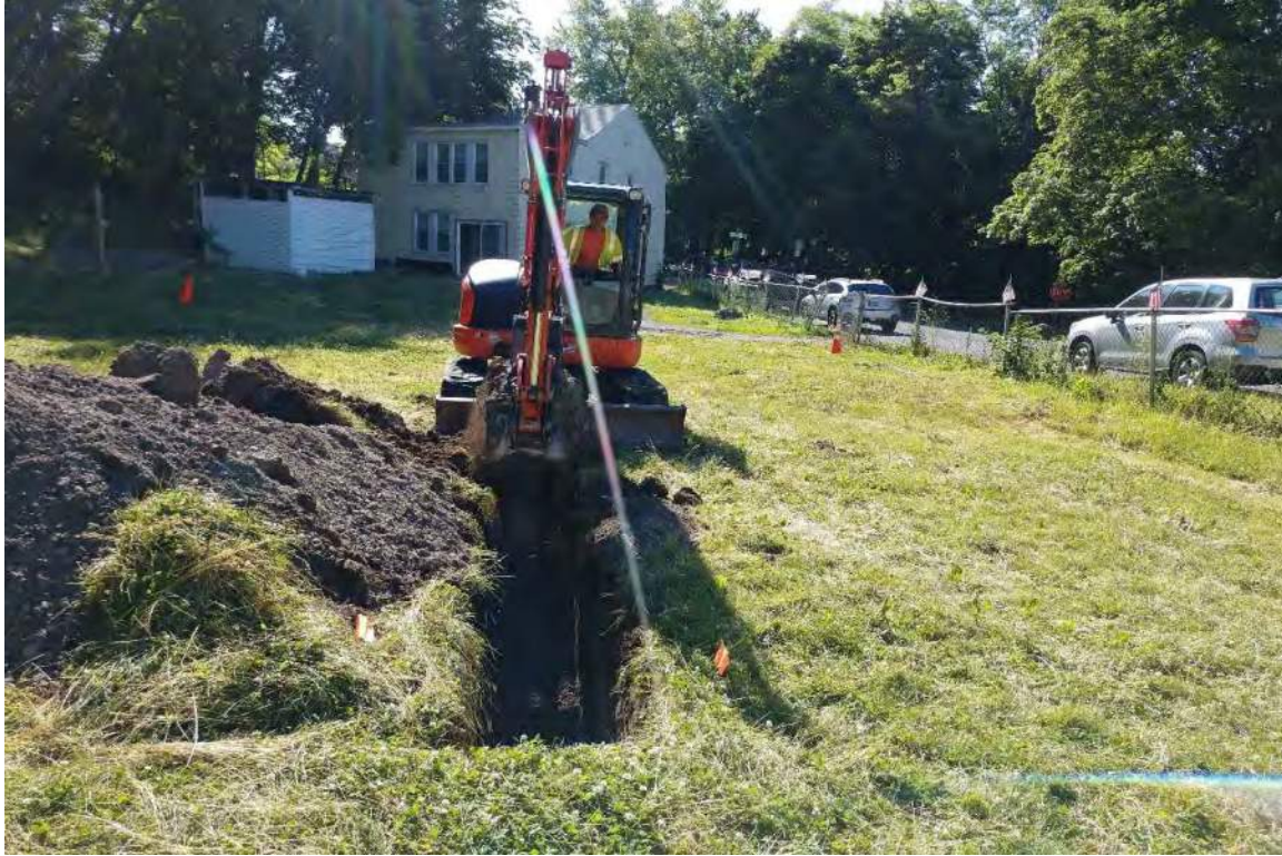
Photo 1: The first trench was completed on the northern side of Scott Street. View to the east.
