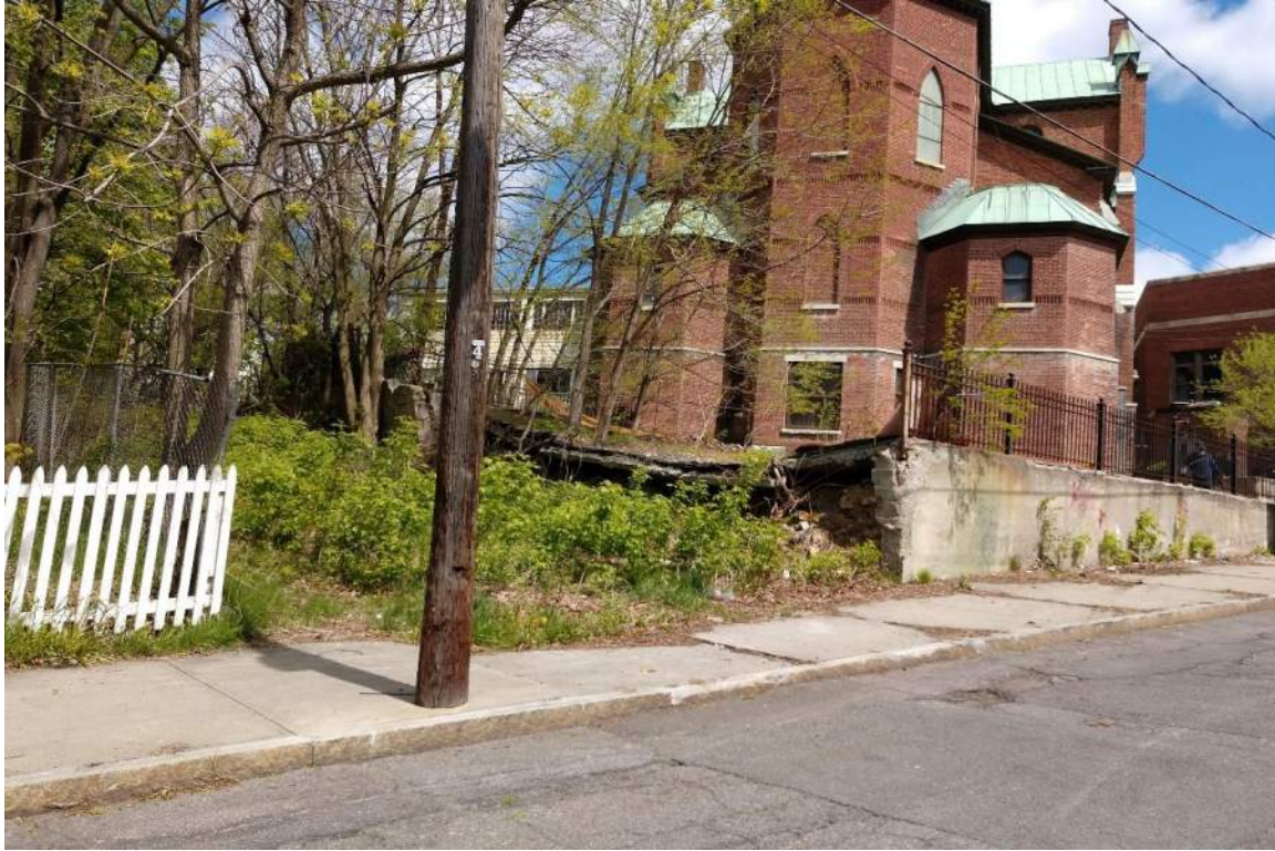
Photo 11: View to the northwest from Krank Street. The retaining wall encloses brick rubble, and portions of brick walls associated with an earlier building.
