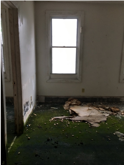
Spreading mold on doorframe, floors, and walls
