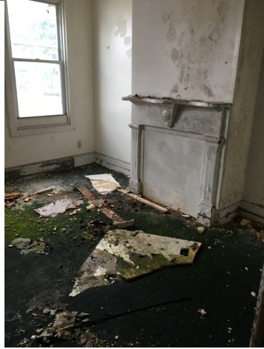
Mold & subfloor rotting in front room
