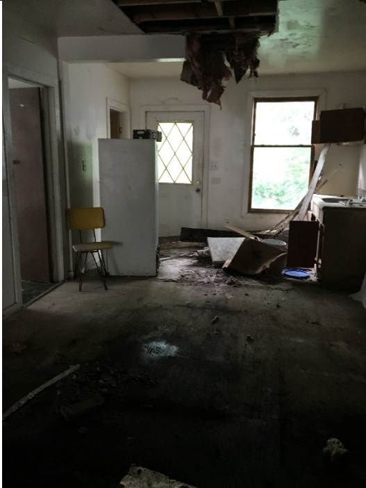
Kitchen, deteriorating ceiling
