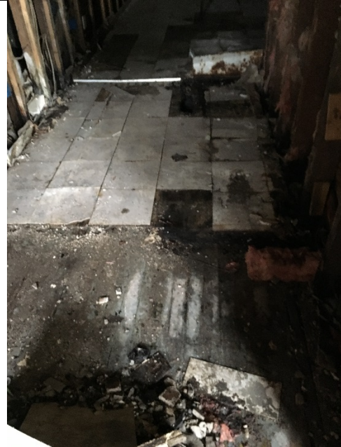
Deteriorating Floor near front entrance
