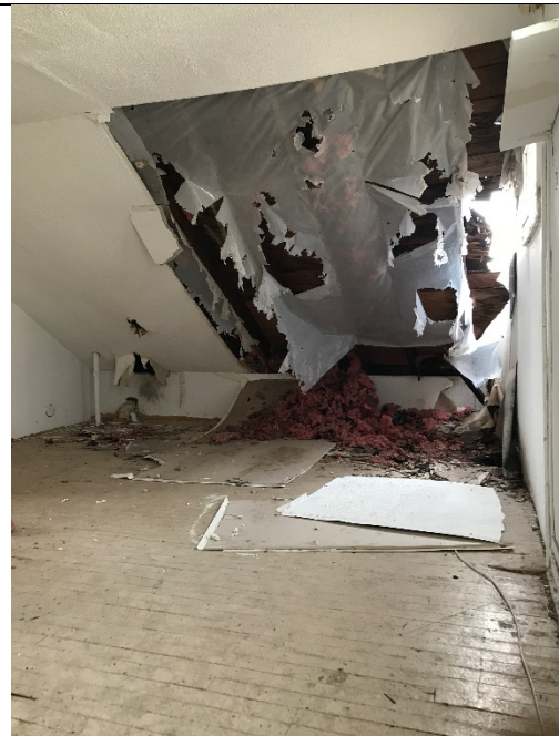
Hole in the attic with evidence of damage from animals in ceiling
