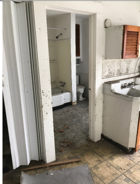
Evidence of mold and water damage on second floor kitchen & bathroom
