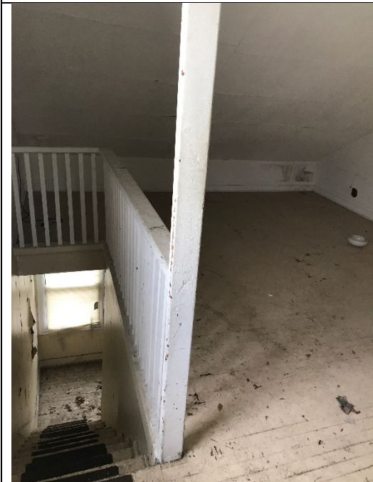
Evidence of water in ceiling causing bowing
