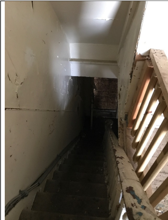
Deteriorating stairs and exposed electric
