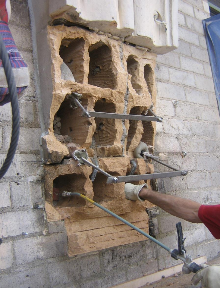
Custom SYSTEM 45 using RL-2 form and pour application at 230 Park Ave, NYC. Anchor system installed into Terra Cotta.
