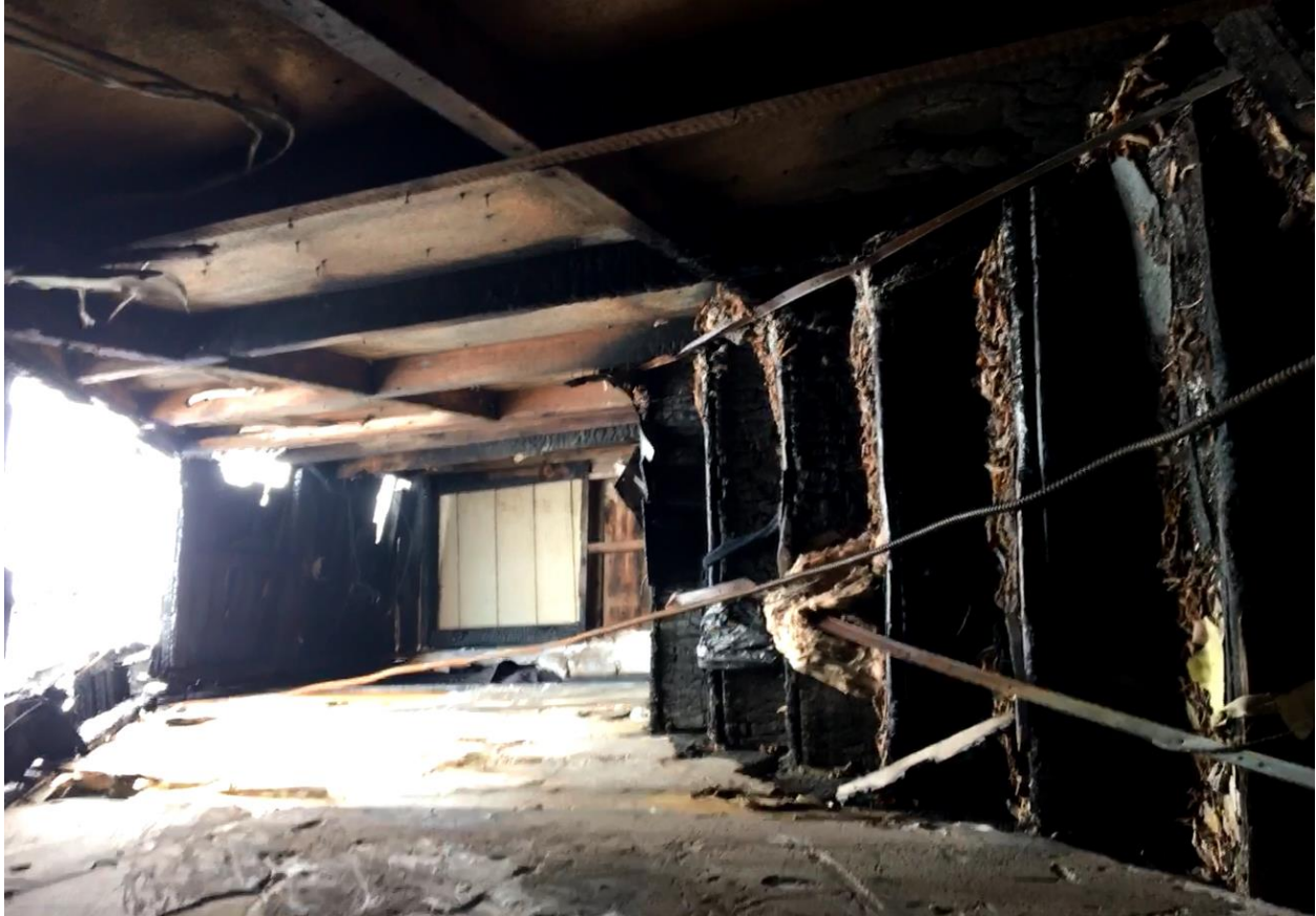
48 Swinton Second Floor. Additional Photos can be found in the Engineer's Report.
