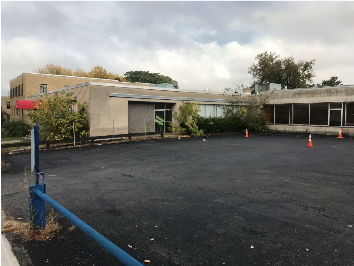
View from South Allen Street of South side of building wing to be demolished
