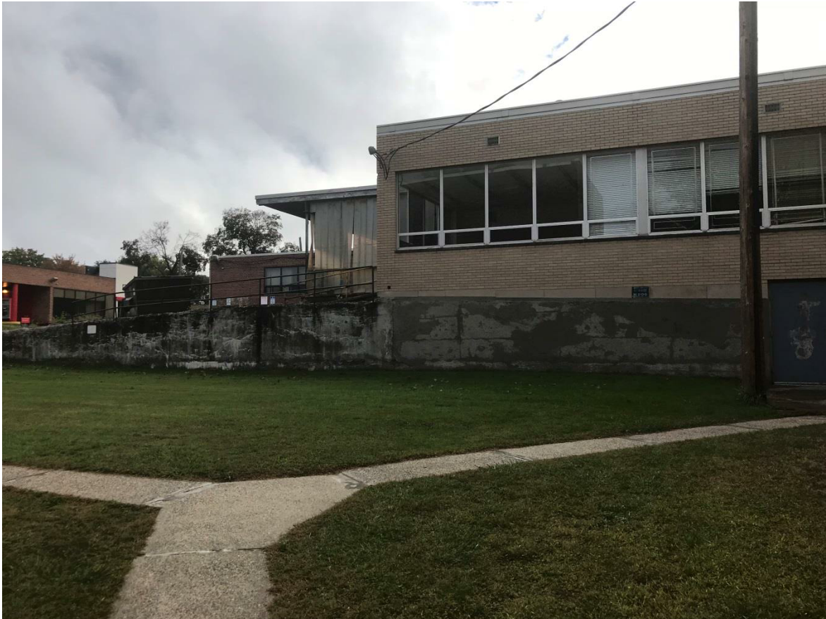
View from rear of North side of building wing to be demolished
