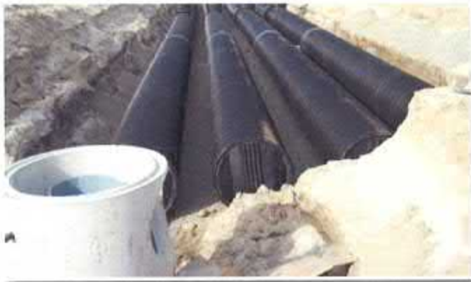
CDS pretreats a rainwater harvesting cistern.
